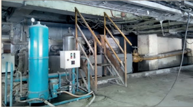
Finish grinding mill No. 1, Gearbox at Lafarge Republic Inc. Iligan Cement Corp. with CJC® Fine Filter HDU 27/108 installed
