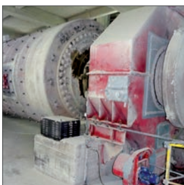
Portlandzementwerk Wittekind with a CJC® Fine Filter installed at the main gearbox of the cement mill ZM I
