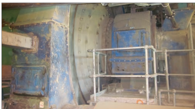
Cement Mill Ireland CJC® HDU 27/54 installed at Trunnion FIXED and FLOATING bearings
