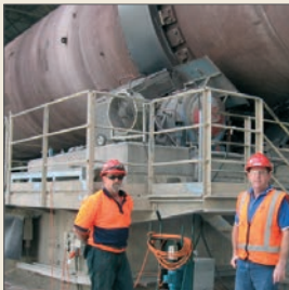
Mr. Phil Immes & Mr. Brad Lewis Golden Bay Cements Rotary Kiln with CJC® HDU 27/27 Mobil Fine Filter installed
