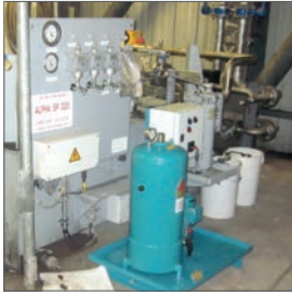
Gearbox, MAAG Gear with installation of a CJC® Fine Filter HDU 27/54 PV
